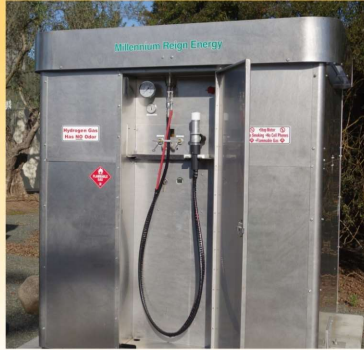
Hydrogen fueling station
